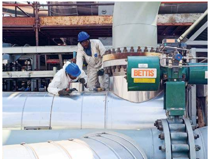
Technicians secure aluminum jacketing on insulated process piping, ensuring full compliance with international thermal performance standards.
