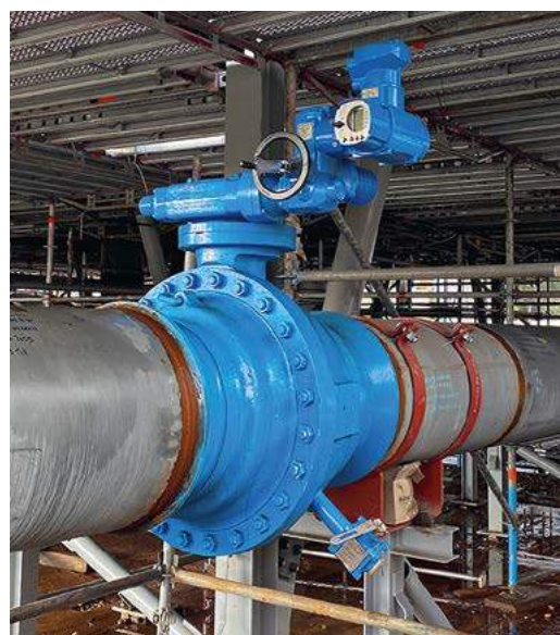
In total, 2,000 Ballostar ball valves have been installed at the CHP plant in Hamburg, Germany.
